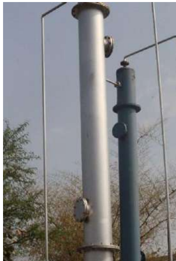
Scrubber Tower at RKDF
