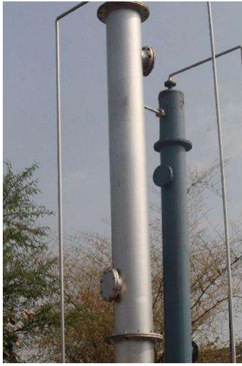
Scrubber Tower at RKDF
