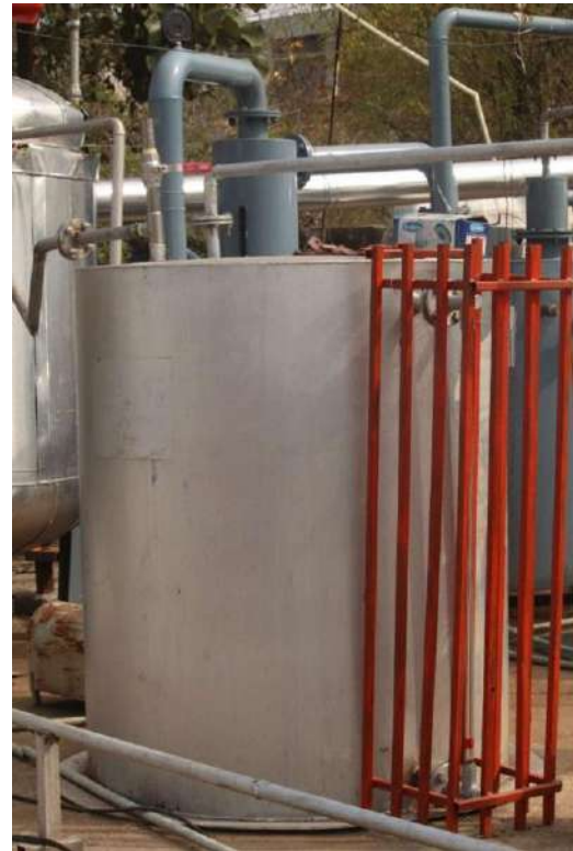
Intermediate Tank at RKDF
